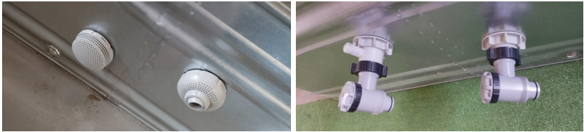
Inlets with valve
